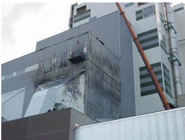
Figure 5 The precipitator after the fire.
