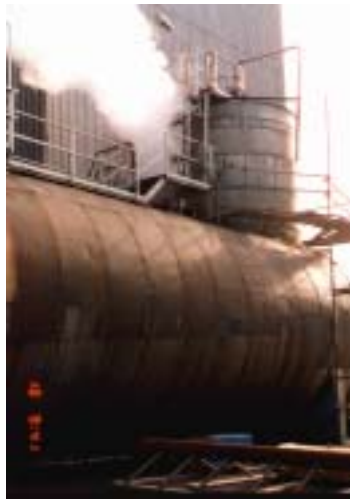
Present situation. Cascade-Type Deaerator
