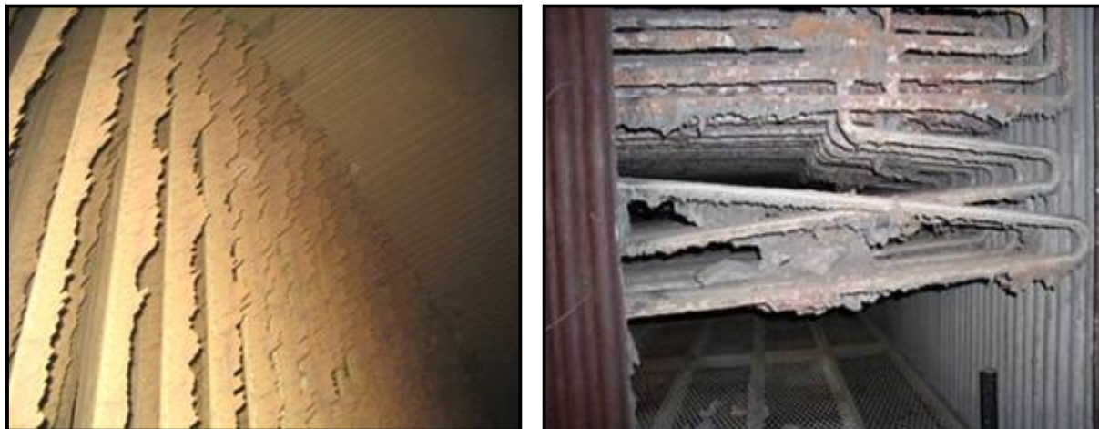
Fouling and corrosion at the superheaters
