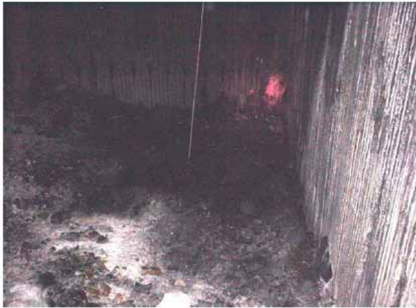
Figure 4, Sodumbikarbonate-cooling caused a small scale smelt-water explosion.
