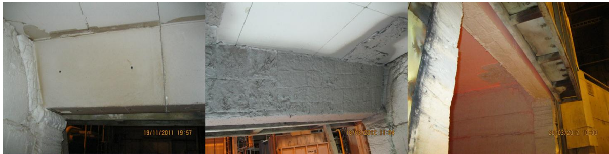
Figure 5. Heat treatment furnace roof protected against heat shocks using veneering.
