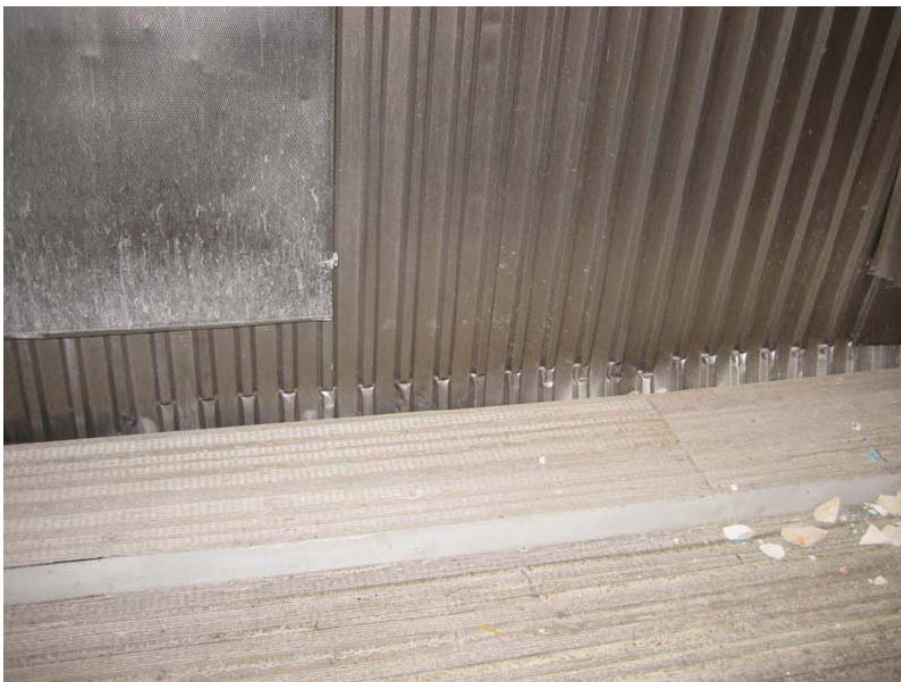
The furnace wall has collided with the platform floor.
