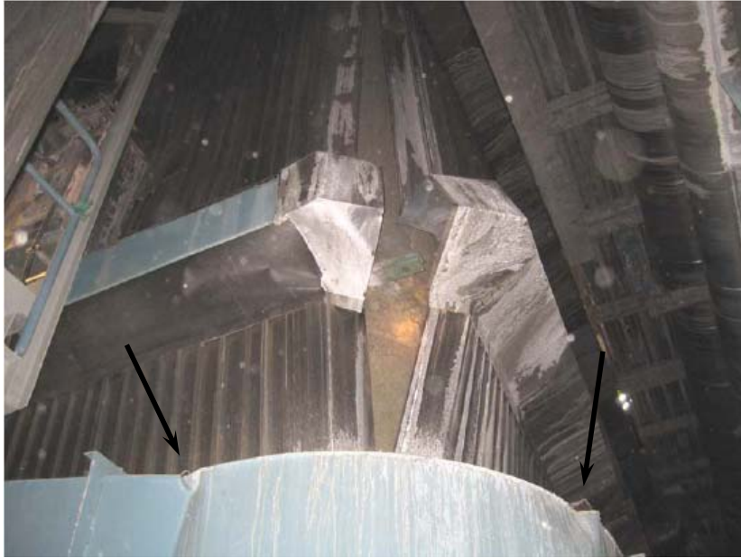
Lagging opened in the boiler's "weak corner". Buck stays have separated, level + 27 m (split pins broken). Damaged air duct (arrows).
